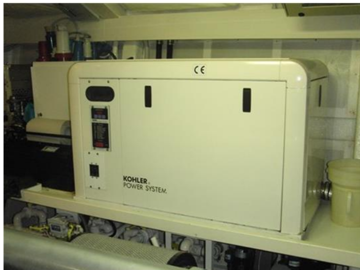
Engine room, Kohler 20 Kw generator, port side
