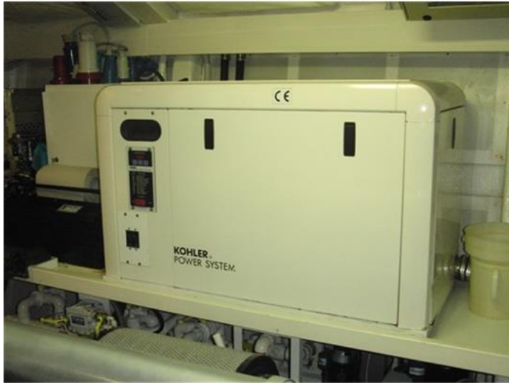
Engine room, Kohler 20 Kw generator, port side
