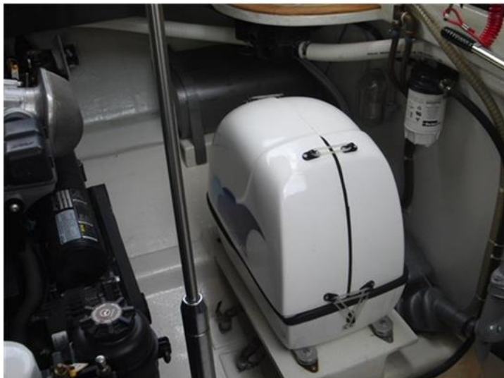
Generator in engine room
