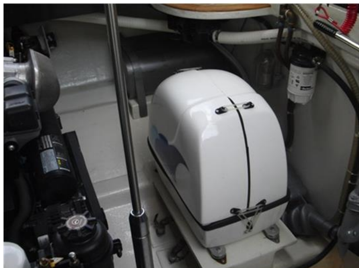
Generator in engine room
