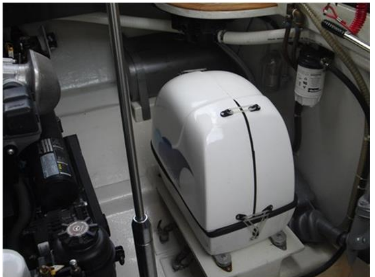
Generator in engine room
