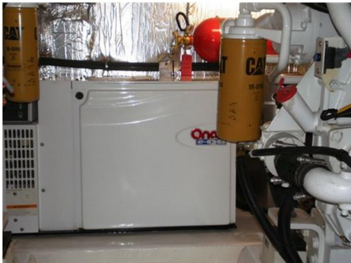
Engine room, generator
