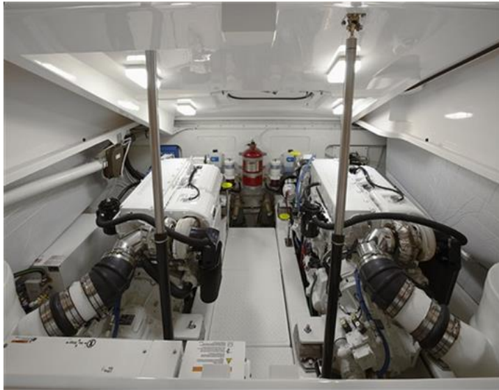
Sistership, engine room
