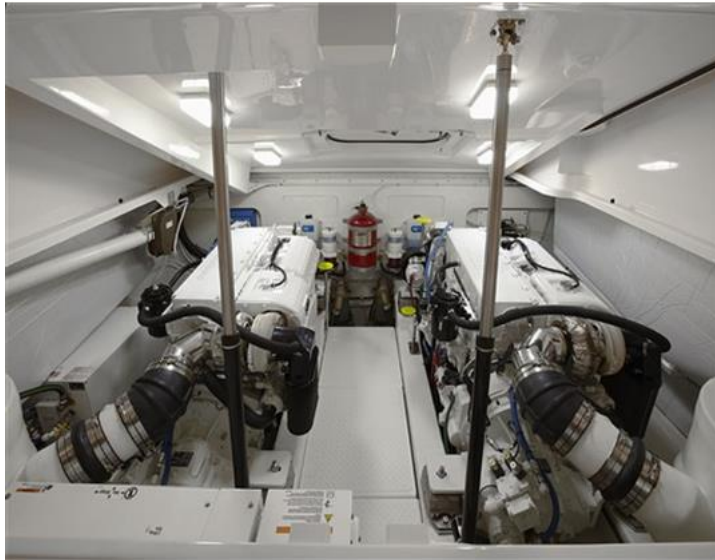
Sistership, engine room
