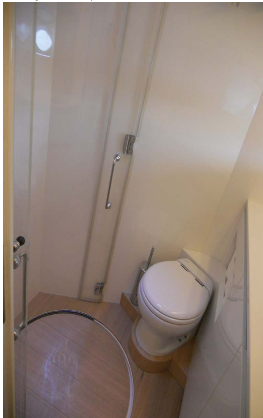
Bagno cabina ospiti - Guest cabin's bathroom
