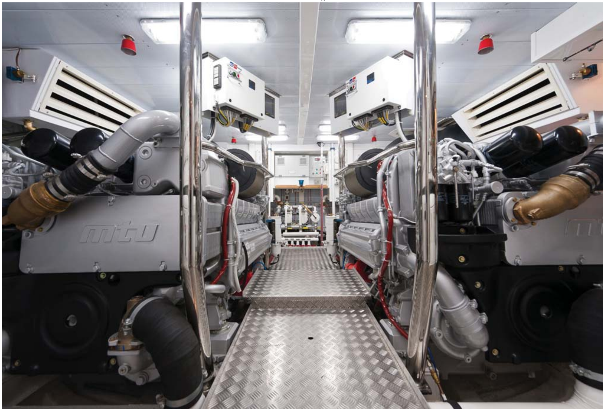
Sala machine - Engine room
