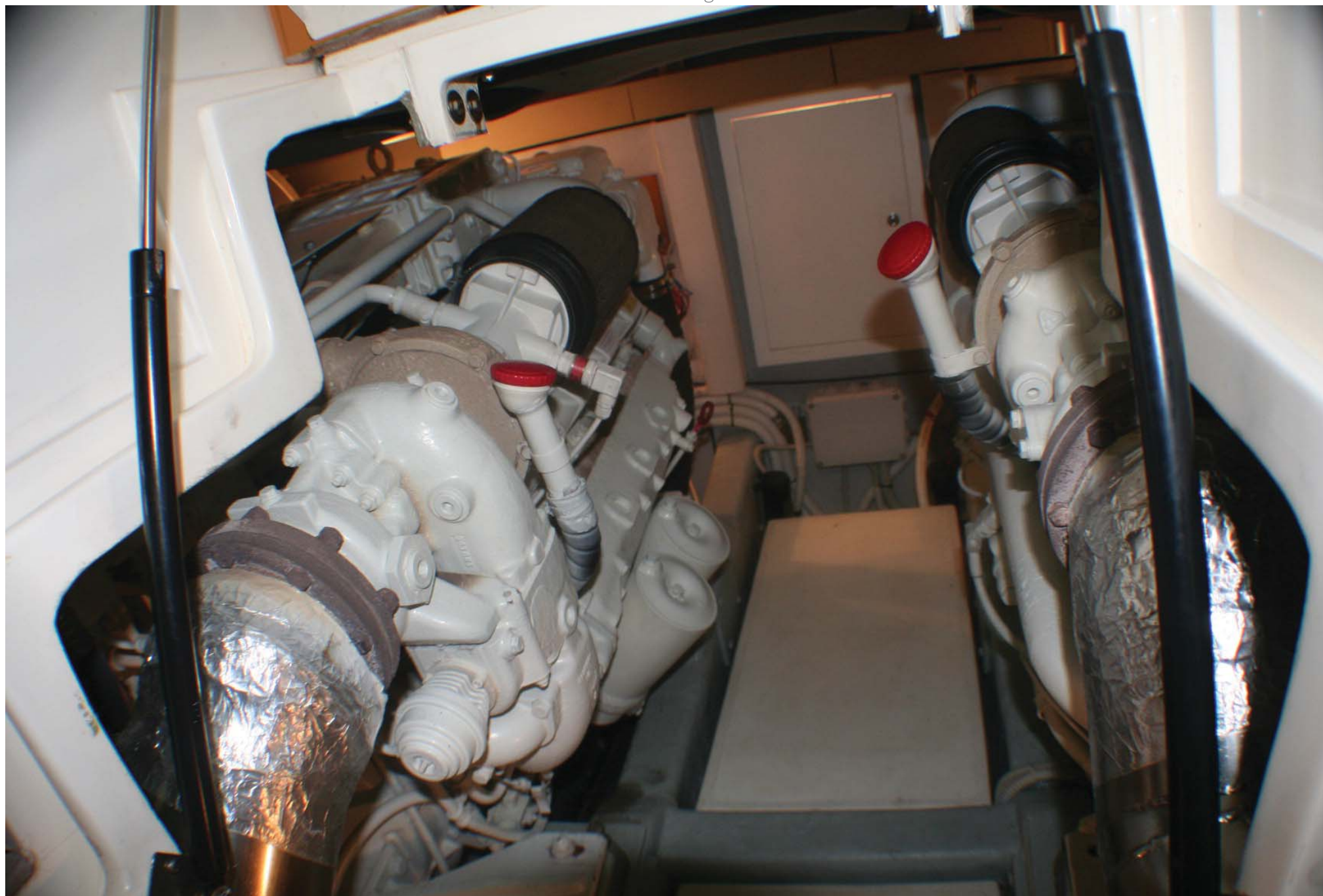
Sala macchine - Engine room
