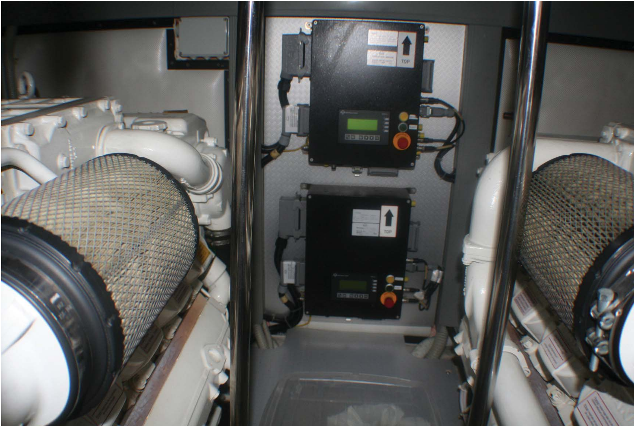
Sala machine - Engine room
