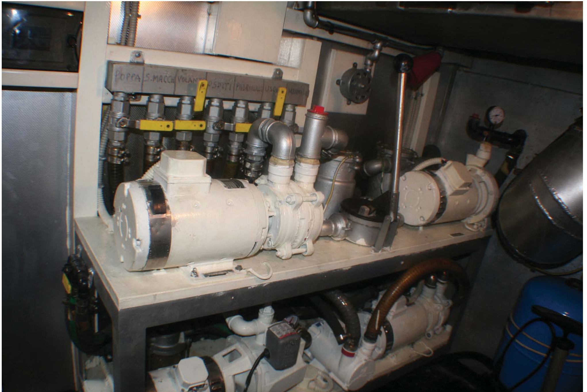
Sala macchine - Engine room
