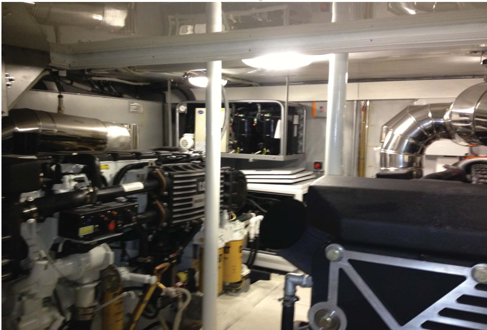
Sala macchine - Engine room
