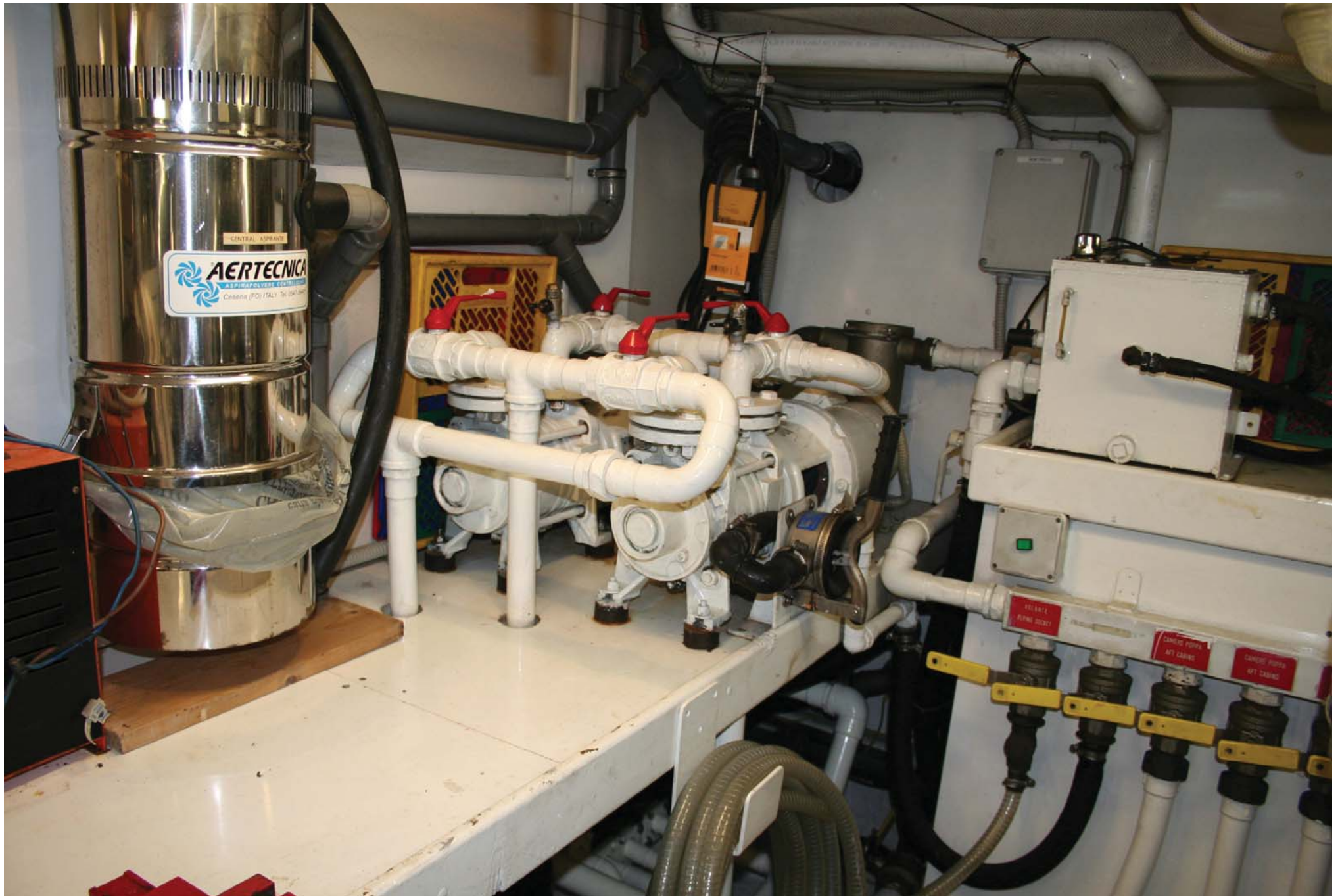
Sala macchine - Engine room
