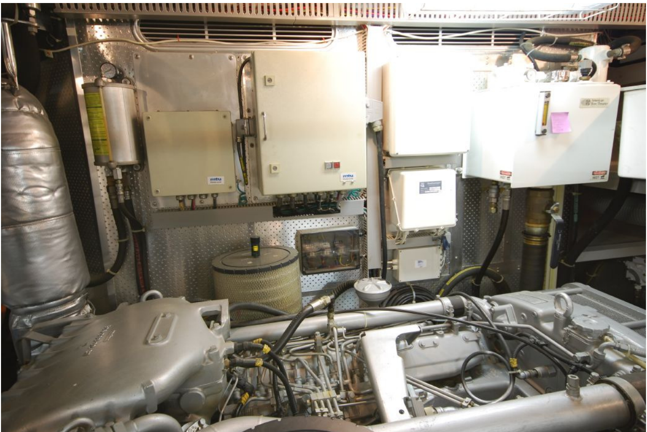
Engine room particular
