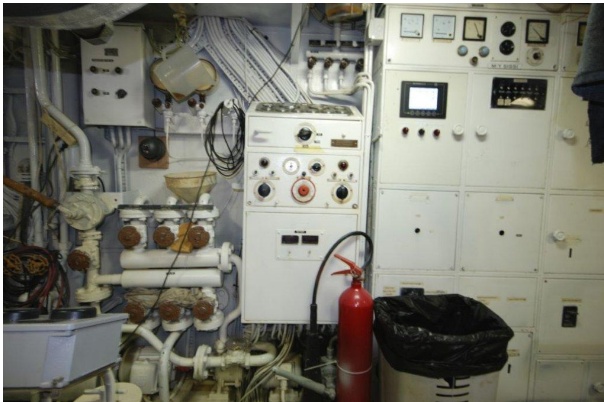
Detail of the engine room
