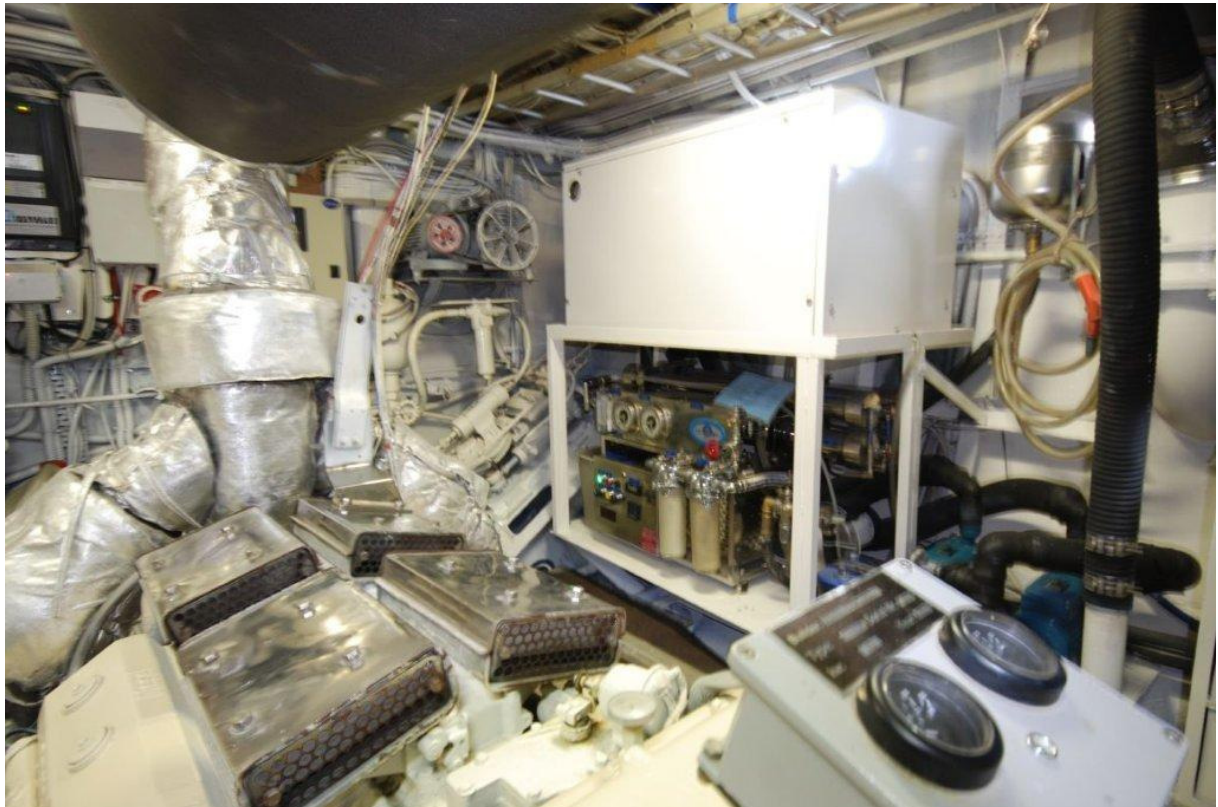
Air conditioning group and watermaker
