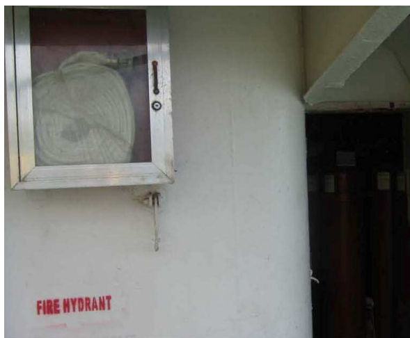
Fire Fighting Equipment
