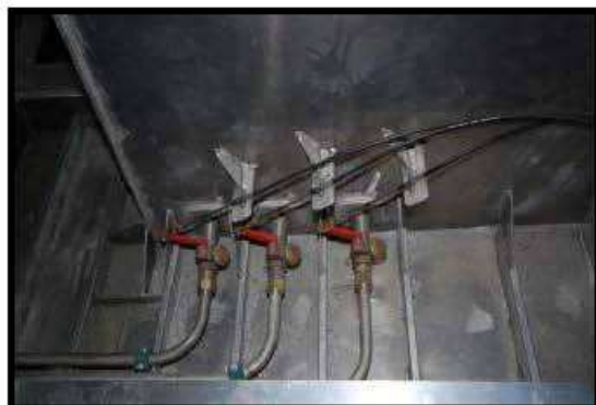
Emergency fuel shut off
