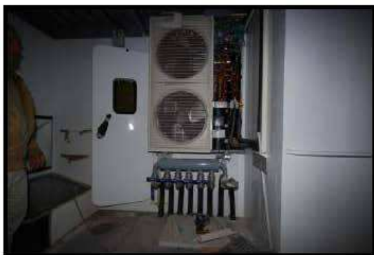
Refrigeration and bilge
