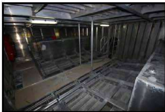
10,000 litres fuel. SS lines
