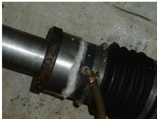
Photo 21 : joint PSS, corrosion
